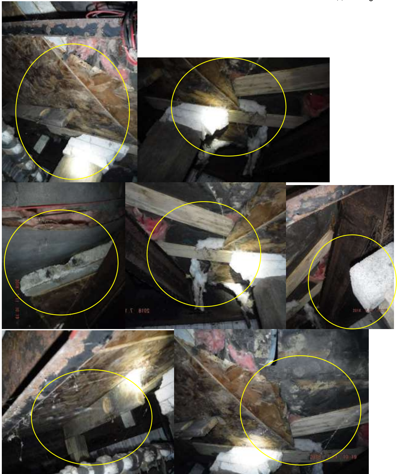
Figure 9 Examples of damaged sub flooring and/or floor joists/structure, dark mold like substances, shimmed with pieced or lumber or boards where sagging, etc.; structural concerns/defects.
