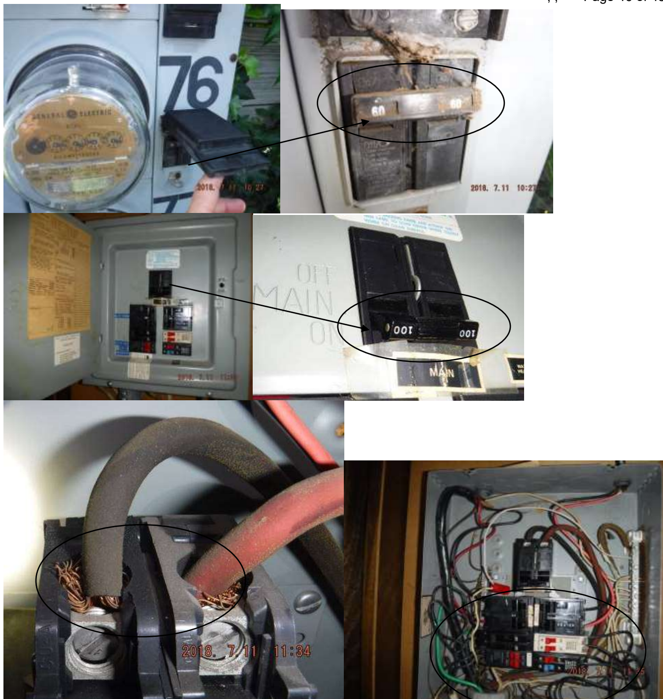
Figure 10 Sub panel was installed unconventional electrical practices; safety concerns.
