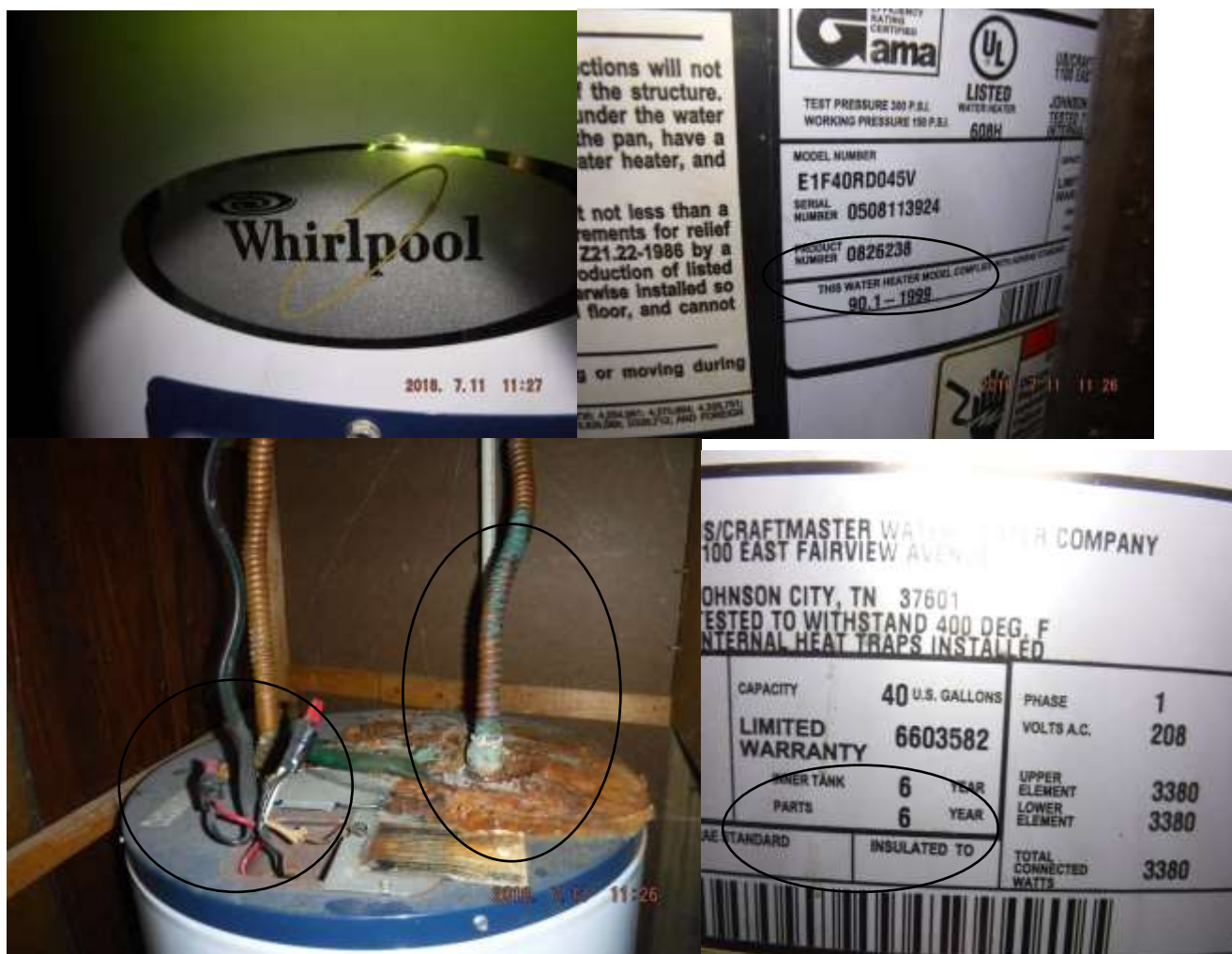
Figure 7 Whirlpool electric water heater in poor condition; electrical wires not recessed in top & covered ( shock hazard), heavy corrosion on tank, flexible water lines & BX wiring
