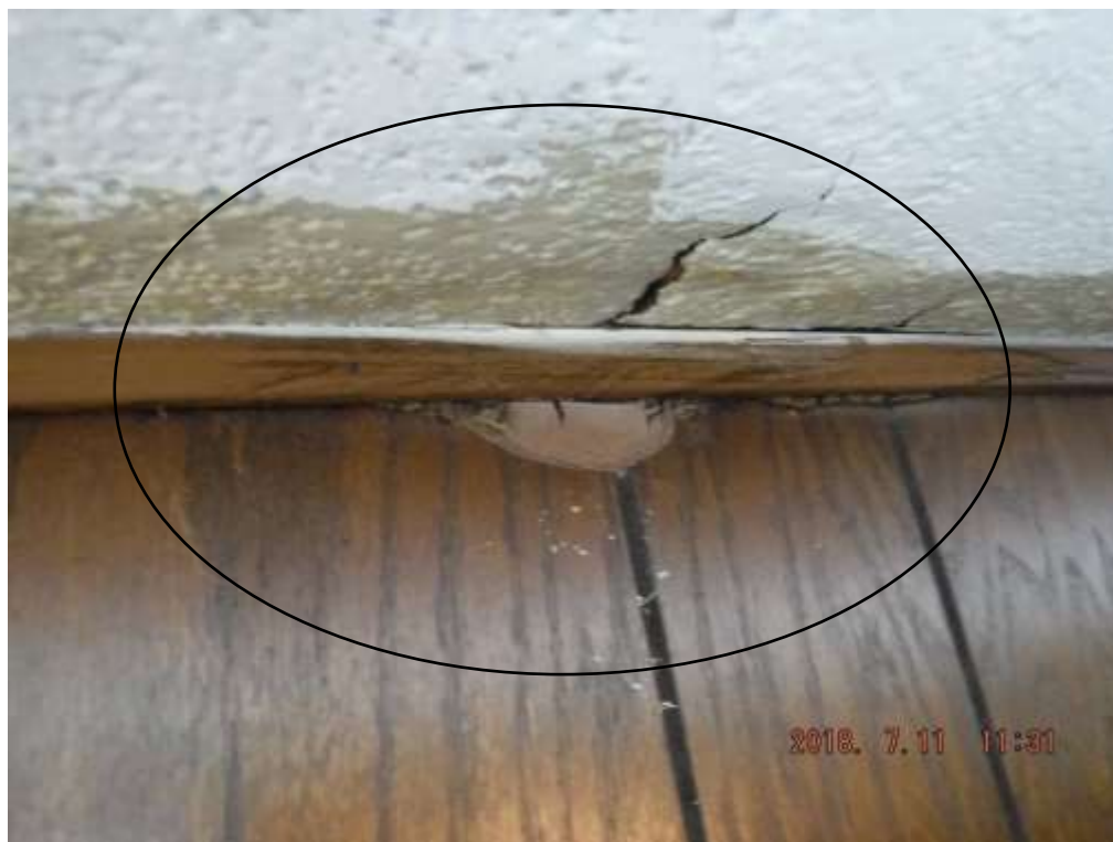
Figure 4 Water damage on ceiling/wall; see roof & exterior section comments.
