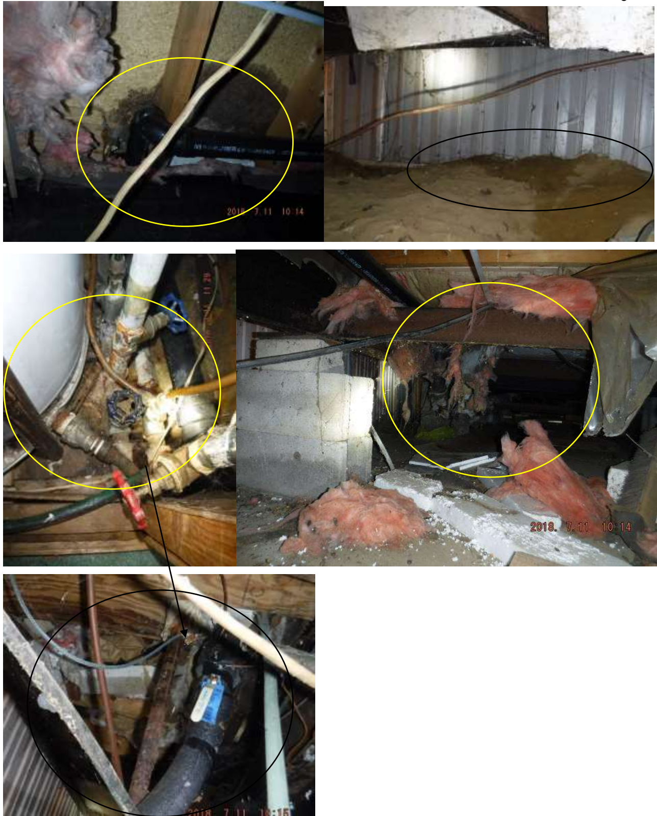
Figure 5 Examples of leaking/corroded plumbing and water stains & damage under the home on subflooring, insulation and fiberboard coverings. Mice droppings visible under home and in side home. Have all damaged repaired, holes sealed and plumbing repaired/replaced.
