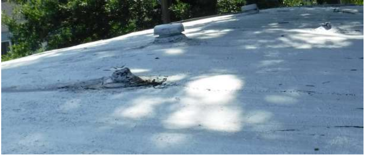
Figure 8 Very short plumbing vent(s); have plumbing vents and the air admittance valve (AAV) evaluated by a licensed plumber & advise on repairs and if AAV allowed by local authorities.
