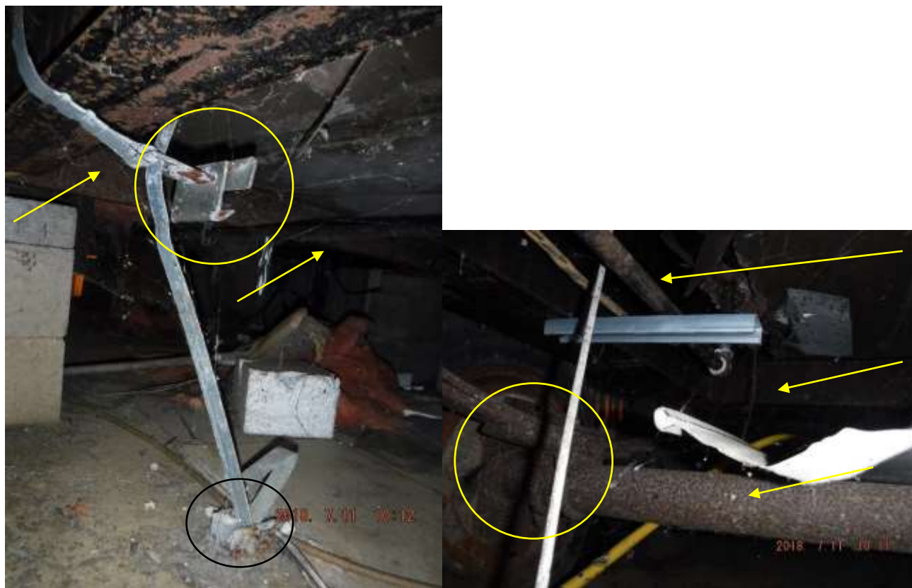
Figure 1 Examples of rust/corrosion, anchors not attached, loose or slack on tie downs, chassis/frame, wheels/axels, etc. Recommend having all anchors & tie downs evaluate/corrected or replaced where needed.
