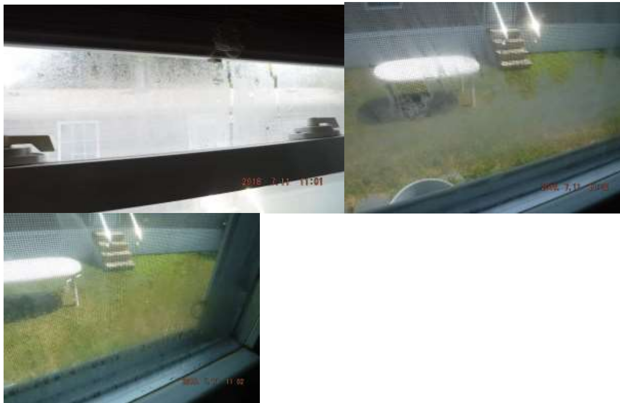
Figure 3 Example of vapor seal breaks; recommend replacing window in the home. See window section comments.
